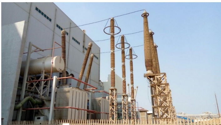
400 kV Power Transformer – RTV coated Polluted Bushings/Insulators (Location: Ras Girtas Power Co., – Ras Laffan C IWPP - Qatar).
